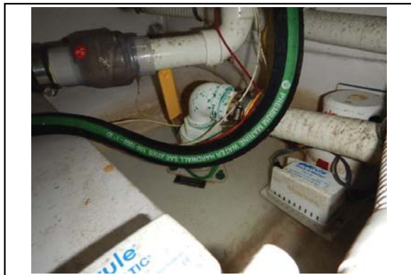
DISCHARGE SEACOCK FROZE
