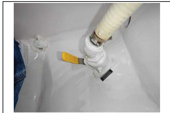
DISCHARGE SEACOCK FROZE
